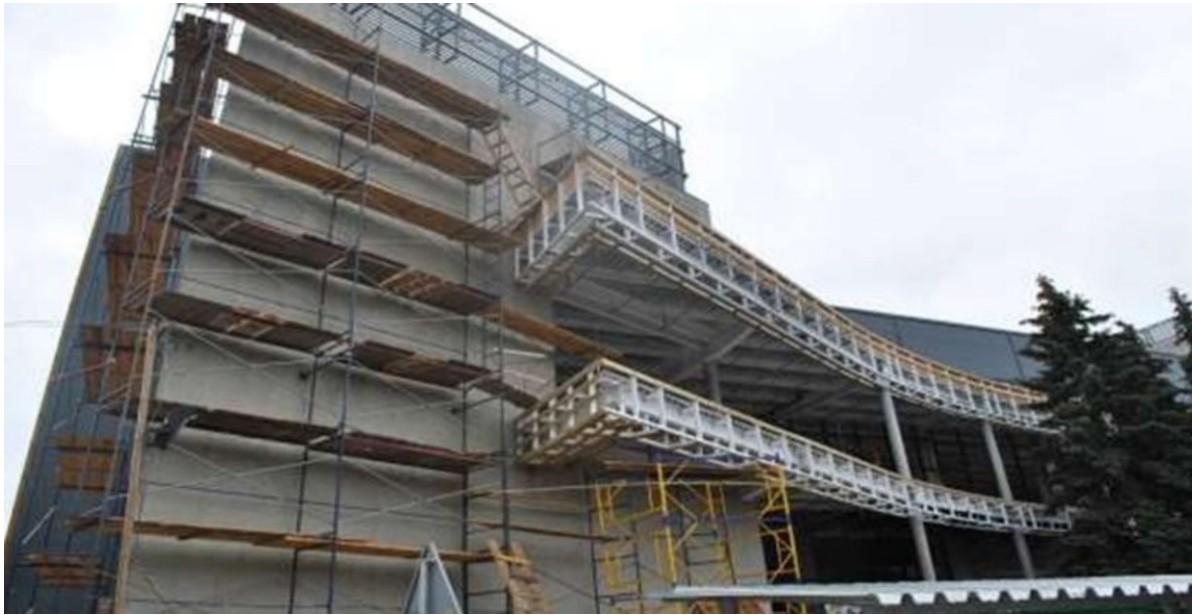
Figure 18 The use of steel-reinforced concrete floors with external reinforcement of profiled sheeting with stampings.
